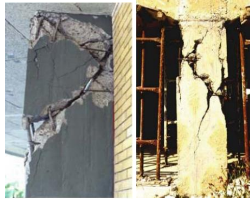
Fig. 1. Shear failures of columns [6]
