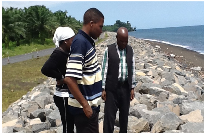
Figure 5. Ripraps which are boulder accumulations have been used along the Limbe Coastline against Coastal Marine Erosion originating from sea level rise
