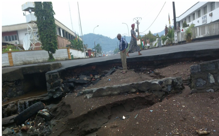
Figure 2. Marine Erosion of the Coastal Highway around BEAC, Down Beach Limbe. Part of the tarred road has collapsed under the impact of the rising sea level
