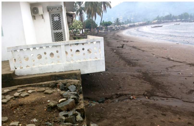
Figure 4. Rising Sea Level and the undermining of built-up structures along the Down Beach Coastline in Limbe
