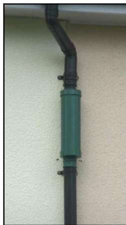
A) Chamber connected to downpipe
